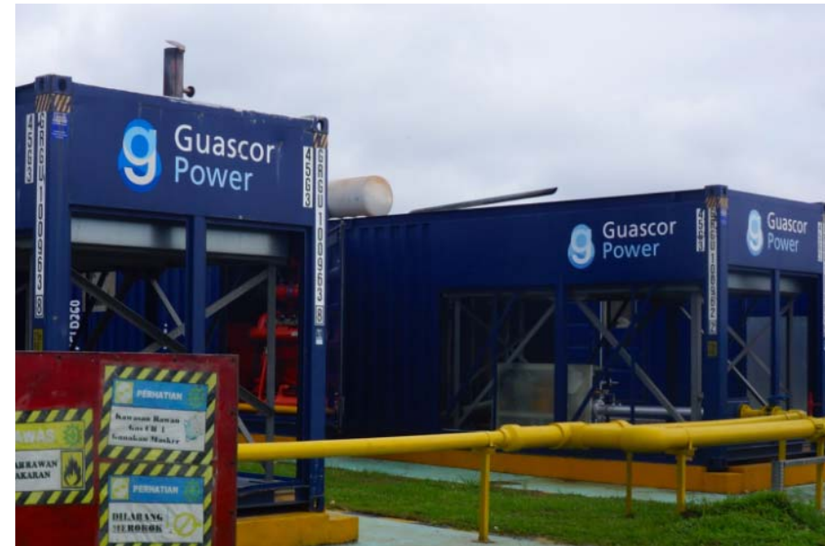
Our Closed biodigester facility at Sei Pelakar Mill, Jambi.
